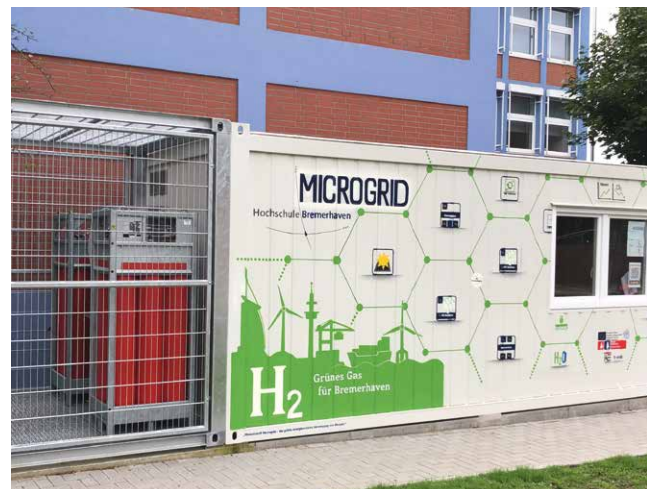
Microgrid container of Bremerhaven University of Applied Sciences
